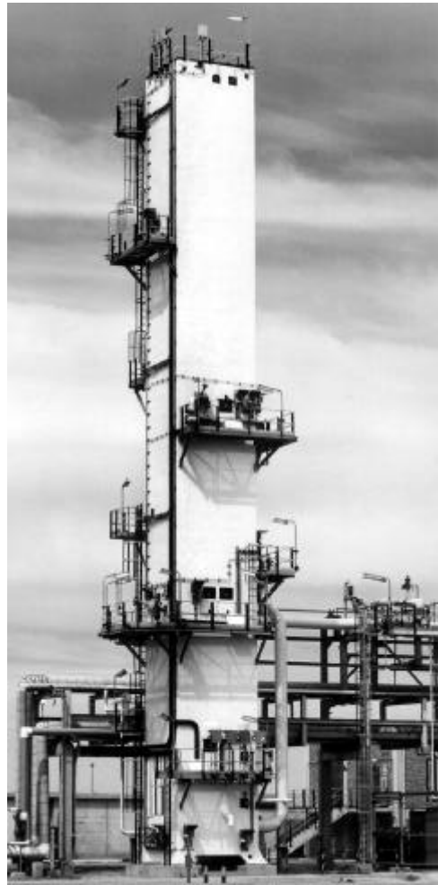
Fig.10: The Mossgas SWHE Cold Box
